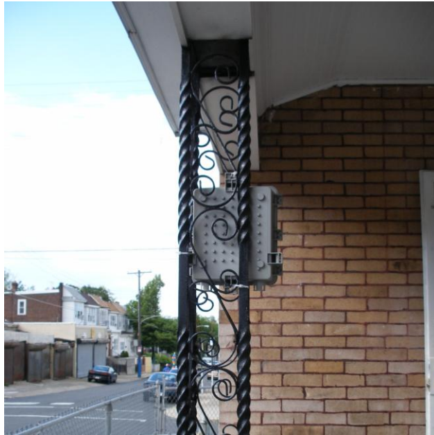
FIGURE 4: SENSOR NODE HUNG ON FRONT PORCH OF HUNTING PARK HOME
